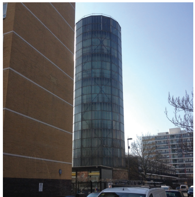
Figure 19. The Thermal Store at Pimlico District Heating Undertaking
