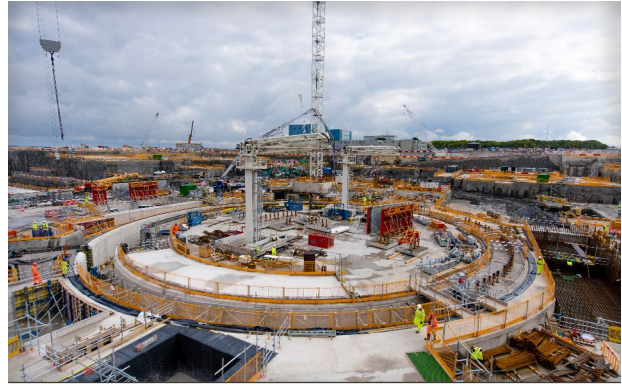
Figure 1. Hinkley Point C nuclear power station construction site in Somerset, South West England, built by EDF Energy
